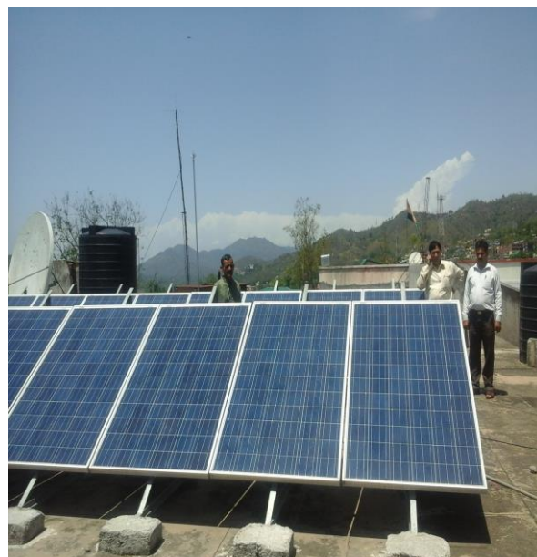
4 kW Solar PV Array at DC Office Bilaspur
