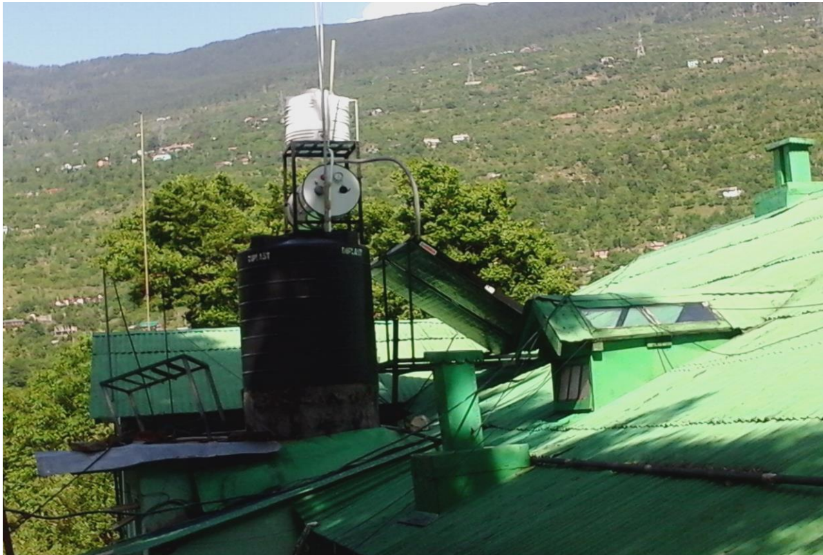
Solar Water Heating System of 200 LPD installed at DC residence, Kullu
