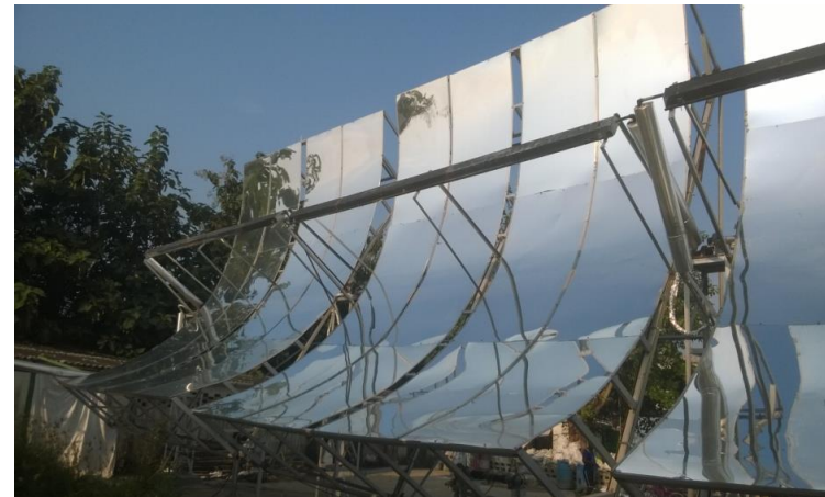
Parabolic Trough Collectors at Siddhartha Surgical, Vadodara (263 m 2 ; Process Heating)
