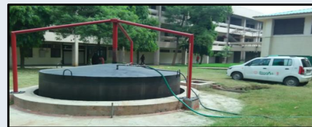
Biogas production, enrichment and bottling facility at BDTC IIT Delhi.
