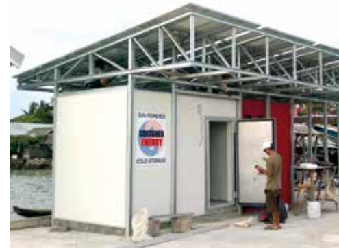
⚡ Solar powered cold storage system
