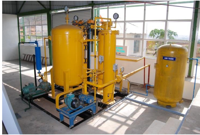
Biogas purification system (PSA Technology) at vill. - Talwada, Taluka - Trimbakeshwar, Dist. - Nasik (Maharashtra)
