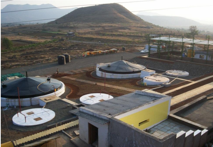
Biogas bottling project of 500 m 3 /day capacity at village - Talwada, Taluka - Trimbakeshwar, District - Nasik (Maharashtra)
